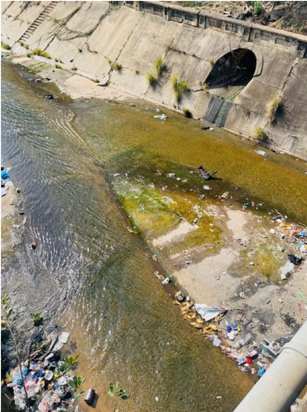
Figure 1: A well-captured picture showing a concrete drainage ditch built stronger to prevent floods, called Lion bridge, filled with stagnant, polluted water, plastic bottles, plastic bags, located at Stanza Bopape Street (Church Street), Arcadia, Pretoria, 0001, on 23 July 2025, 12:51 p.m. It is the oldest existing bridge over the Apies River and replaced an older bridge called Arcadia Bridge [Photographer: Mononela Naniki].
