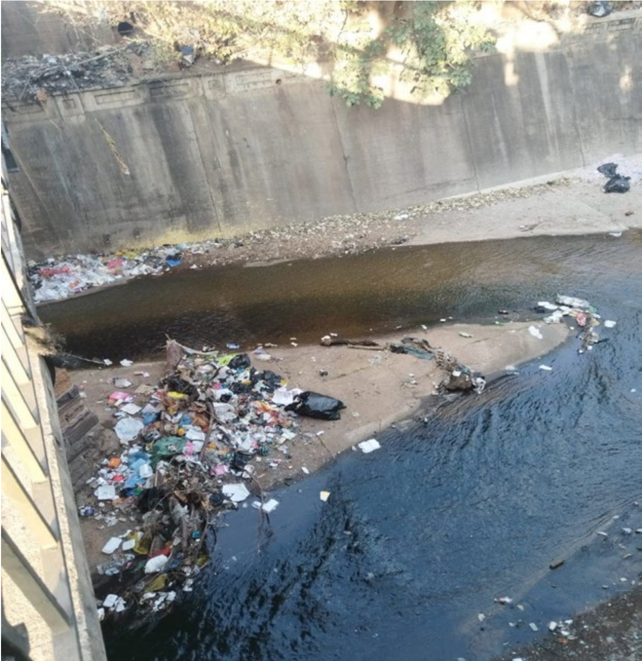
Figure 4: The Walker Spruit river binds with the Apies river in Lions Bridge. This is clearly a run off from the waste of the city down to the canal causing water pollution. The water pollution is carried through out from Sunnyside down to Arcadia it doesn't get any better. A canal beauty lost, overwhelmed by humanity's neglect Taken on the 10 th of August , 2025. (Photo: Melissa A Dlaku)
