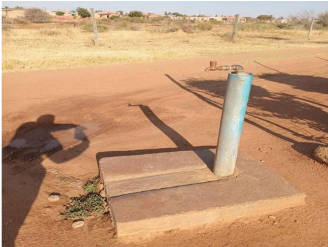
Figure 5: This image shows a tap that has been dry for a few days and it also shows that the tap is not in a good shape, shot by Sethole Khohlisane around 9 th August 2025 at Botlokwa village in Limpopo.
