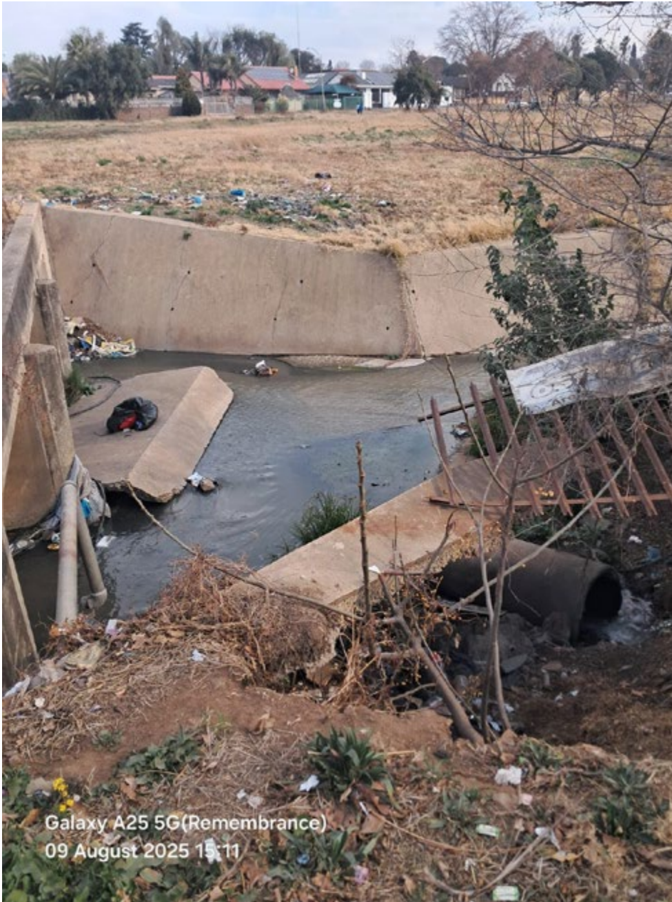
South Africa, Johannesburg Vanderbijlpark, 09 August 2025 taken by Mapoulo K Concrete lined channel filled with water and significant amounts of litter and debris.
