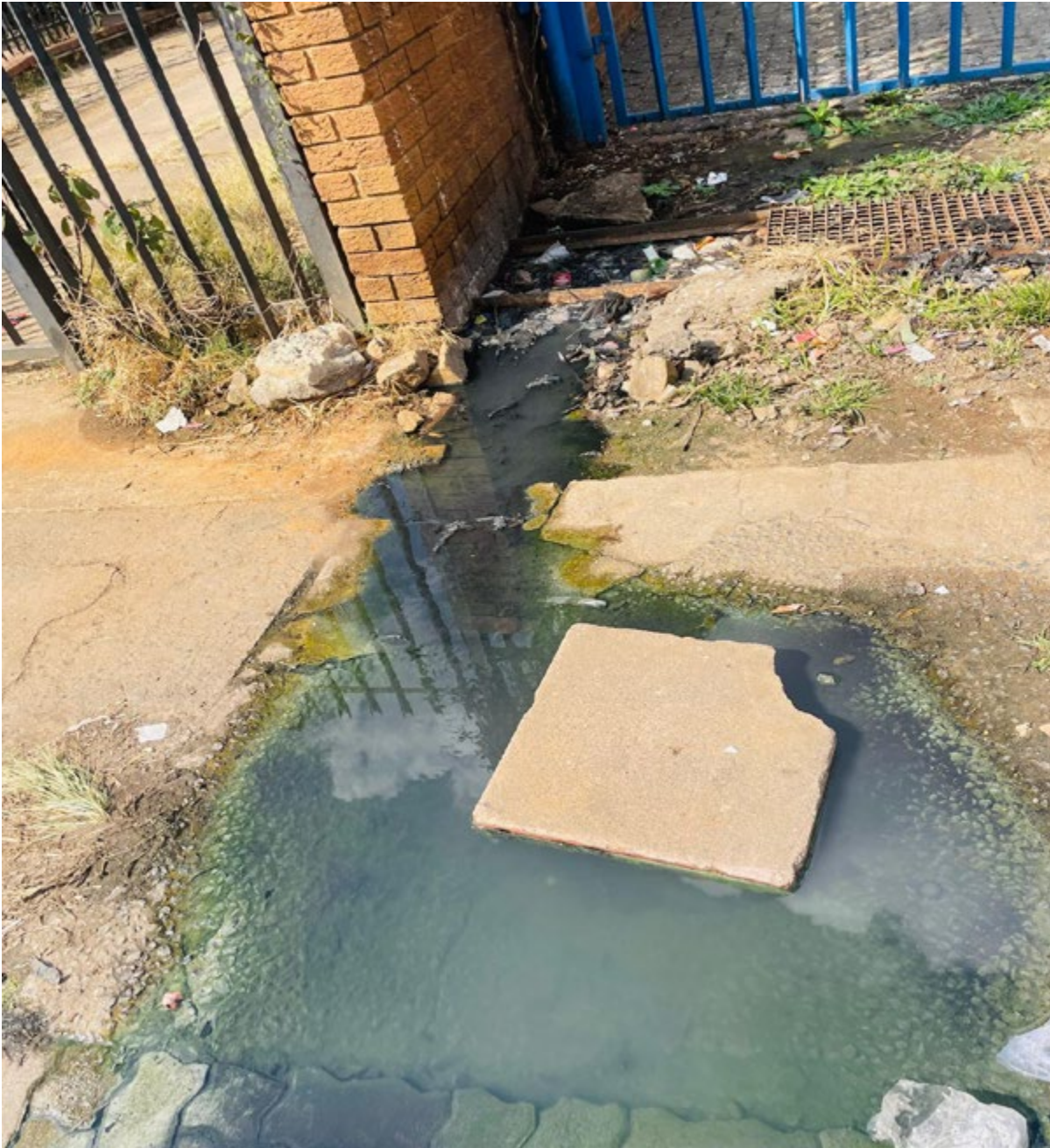
Figure 3: A well-captured photograph showing the overflowing of sewage that contains wastewater from households and businesses near a mall called Sunny Park, located around the corner of Steve Biko Street and Robert Sobukwe Street in Sunnyside, Pretoria, 0002, on 23 July 2025, 1:10 pm [photographer: Mononela Naniki].
