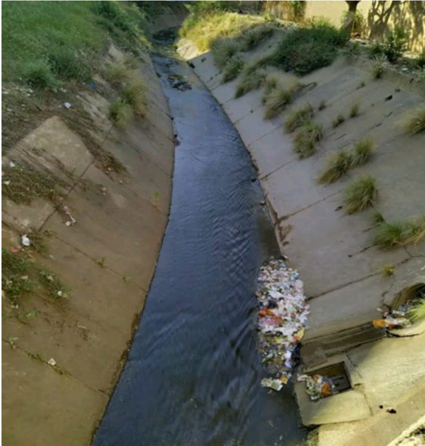
Figure 3: A canal chocked with plastic waste and dirt threatning the environment and animals. The contaminants flows down the Walkers spruit river, blocking the drainage system of the canal too much accumulation of plastic, papers and sweets . Taken 6 August 2025,(Photo: Melissa A Dlaku)
